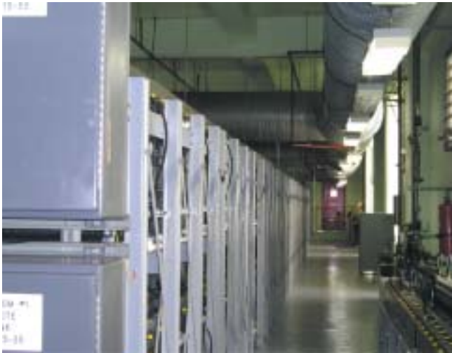
Exhibit 7.4 LA battery rack at PREPA's Sabana Llana BESS (source: PREPA)
