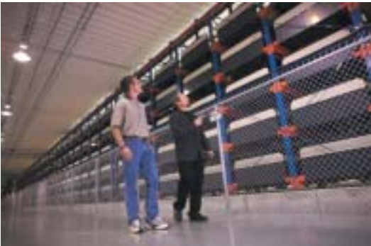
Exhibit 7.8 Ni-Cd battery rack at GVEA's Fairbanks BESS (source: ESA/Saft)
