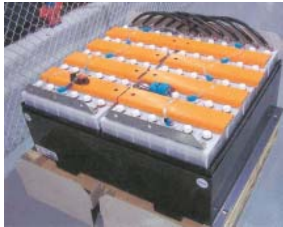
Exhibit 7.9 10-cell Ni-Cd battery module at GVEA's Fairbanks BESS (source: ESA/Saft)
